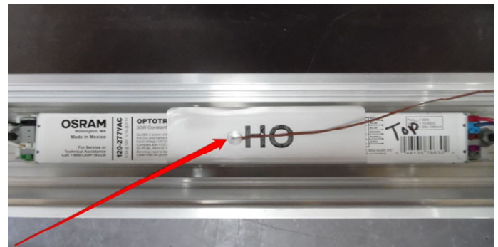
Driver Thermocouple Location 1 (Top)
