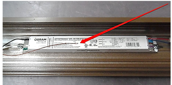
Driver Thermocouple Location
