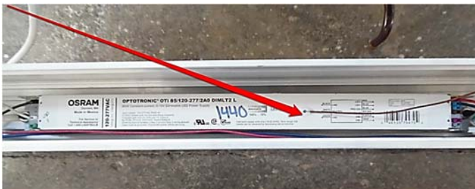
Indirect LED Driver Location 1
