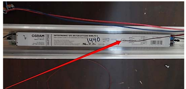
Indirect LED Driver Location 2
