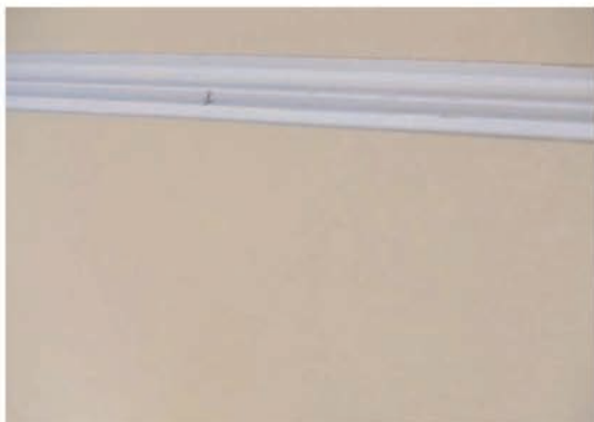
3) The wall is textured and finished, leaving a perfectly straight channel, ready to receive the fixture's reflector assembly.
