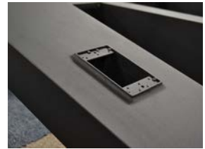
GFCI CFCI Box
